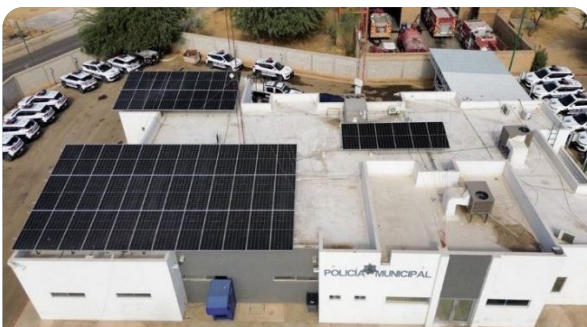
Comandancia El Cortijo gets a clean energy upgrade. Photovoltaic system installed for sustainable power.
