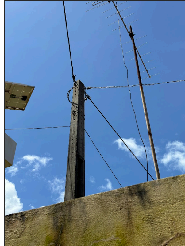
Electrical connection, next to the building
