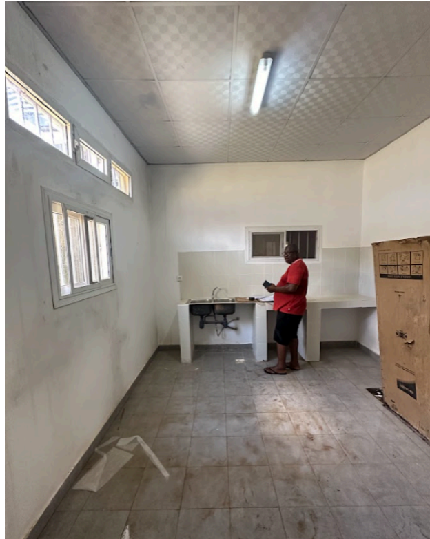
“Copa” room. The room available for being transformed into a cooling chamber
