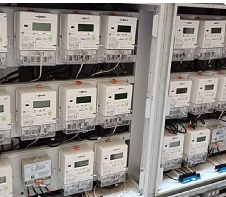
Smart metering setup in Colombia.
